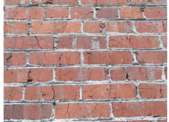
Photo 2- Cracking of bricks
