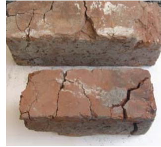
Photo 3- Exterior Cracked Bricks
